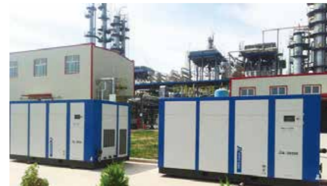
355KW water cooling air compressor in Algeria Chemical Plant
